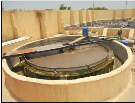
Picture 17: STP Clarifier
