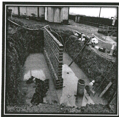
Image 5: Storm water catchment pit 2
