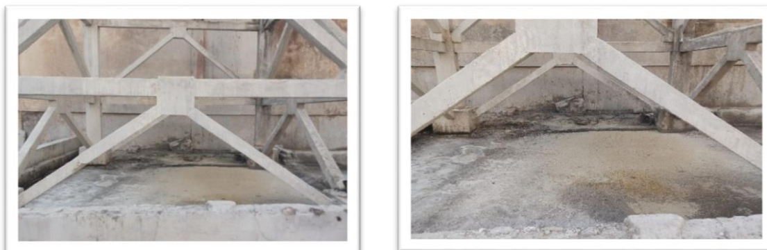
Representative Images of spillage below conveyance system
