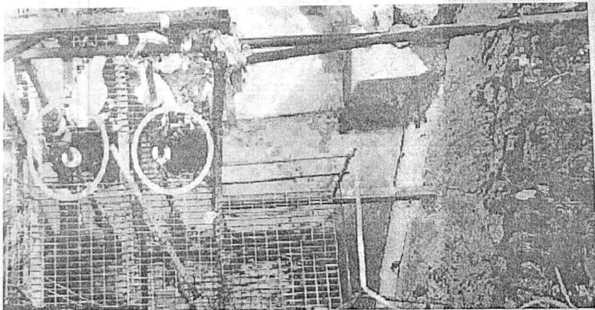
Image 6: Onsite photograph Culvert catchment pit built by the Unit to gather the runoff water and the highlighted two water submersible pumps
